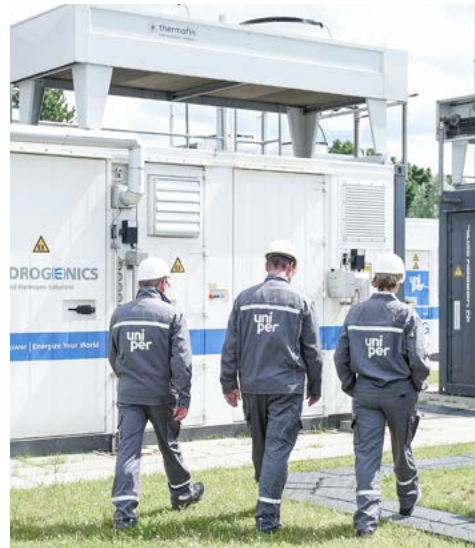
Uniper employees at our power-to-gas unit in Falkenhagen, Germany.
