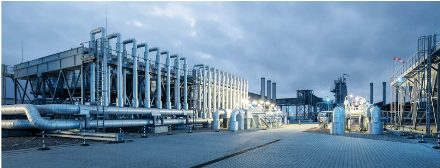
Etzel gas-storage facility in Germany at night.
