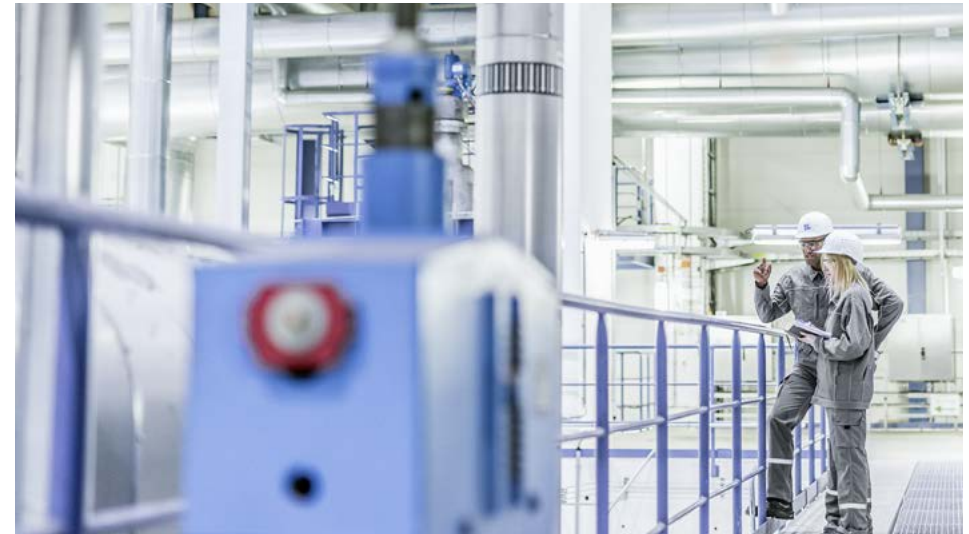
Uniper employees at Maasvlakte power station, Netherlands.
